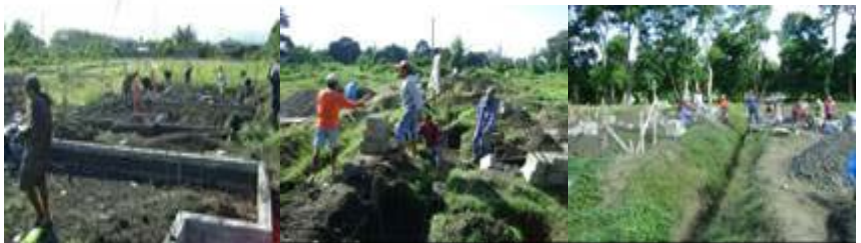
▲ Ground works for the first 18 housing units at the St. Luke Subdivision.
